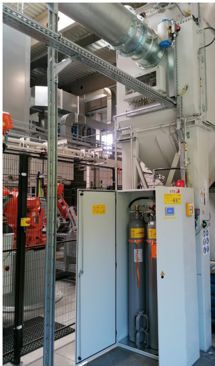
Filter unit with a CO 2 compact fire extinguishing device
