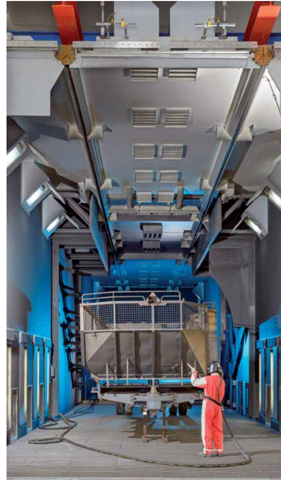
If the turbines did not shot blast some surface areas, these areas can be subsequently shot blasted manually.
