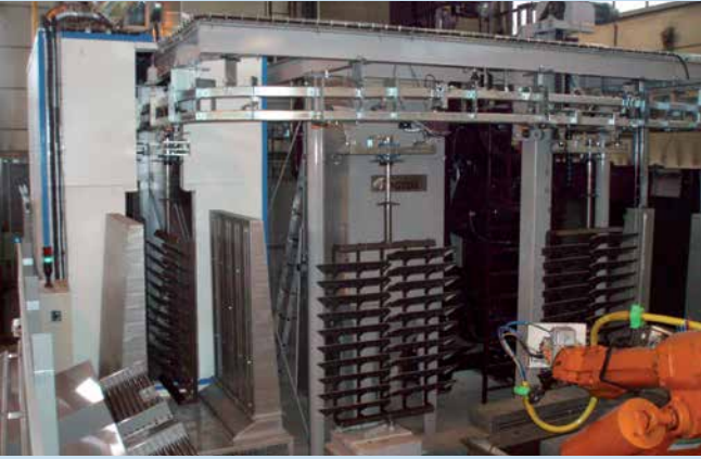
Continuous overhead rail shot blast plant for cleaning blank parts
