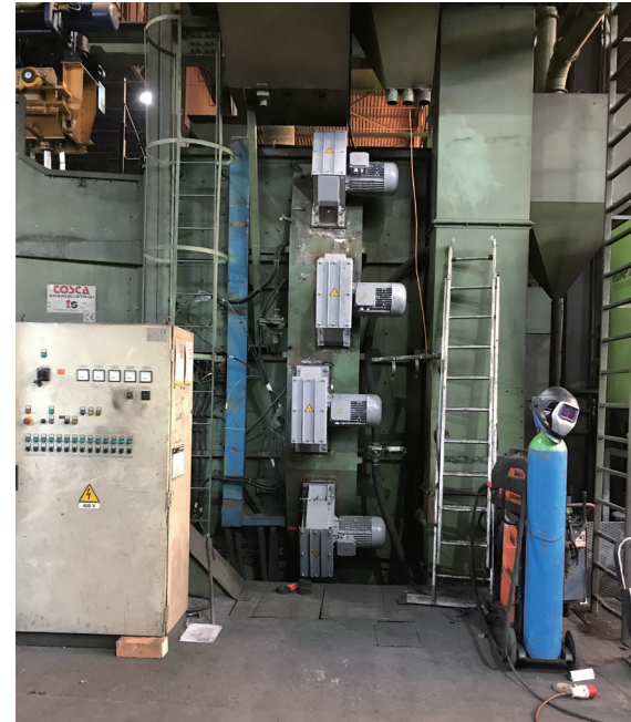
Four new AGTOS high-performance turbines on the modernized overhead conveyor blasting machine
