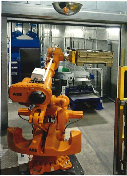
View of the blasting cell, with robot, blasting machine and conveyors
