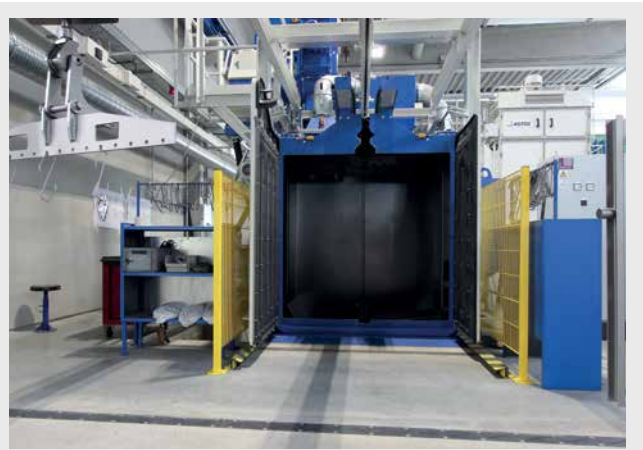
In the AGTOS HT 17-17 type monorail blast machine small parts can be blasted automatically.
